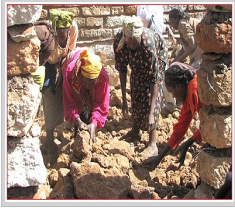
Women from the Kangeta community take turns helping with construction of the new Day Care Centre
