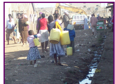
The main roads in Koch are being graded for bitumen, a much awaited improvement to the lives of the people. Structures have to be pulled down to make room for progress.
